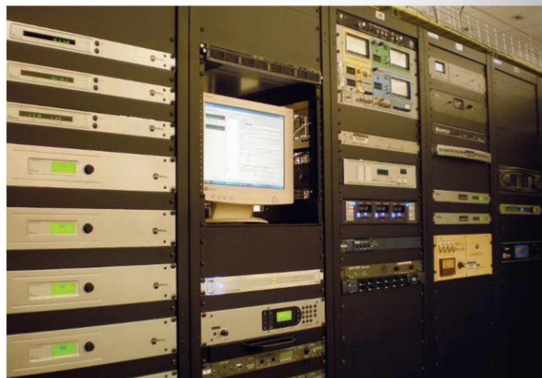
KUNV's rack space in the TOC includes Omnia 6EXi and Omnia One processors, Axia engines and audio nodes, Comrex Access, Arbitron PPM encoders, Public Radio Satellite System hardware, streaming server/encoders and iMediatouch skimmer. Also at work is gear from Sage, Broadcast Tools, DaySequerra, QEI, Orban, Moseley and Belar, among others.
